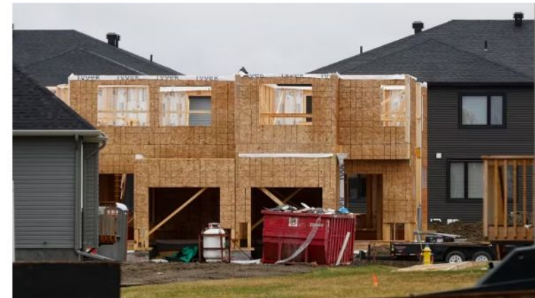
A house is shown under construction in Ottawa in April. With a housing shortage and affordability crisis in Canada, advocates say people with disabilities are contending with less inventory because most units aren't built with accessibility in mind. (Lars Hagberg/Reuters)
